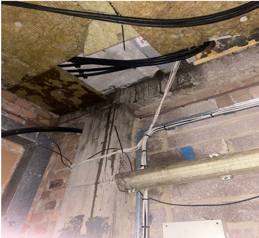
Leaks entering an electrical cupboard from the bathroom of the flat above
