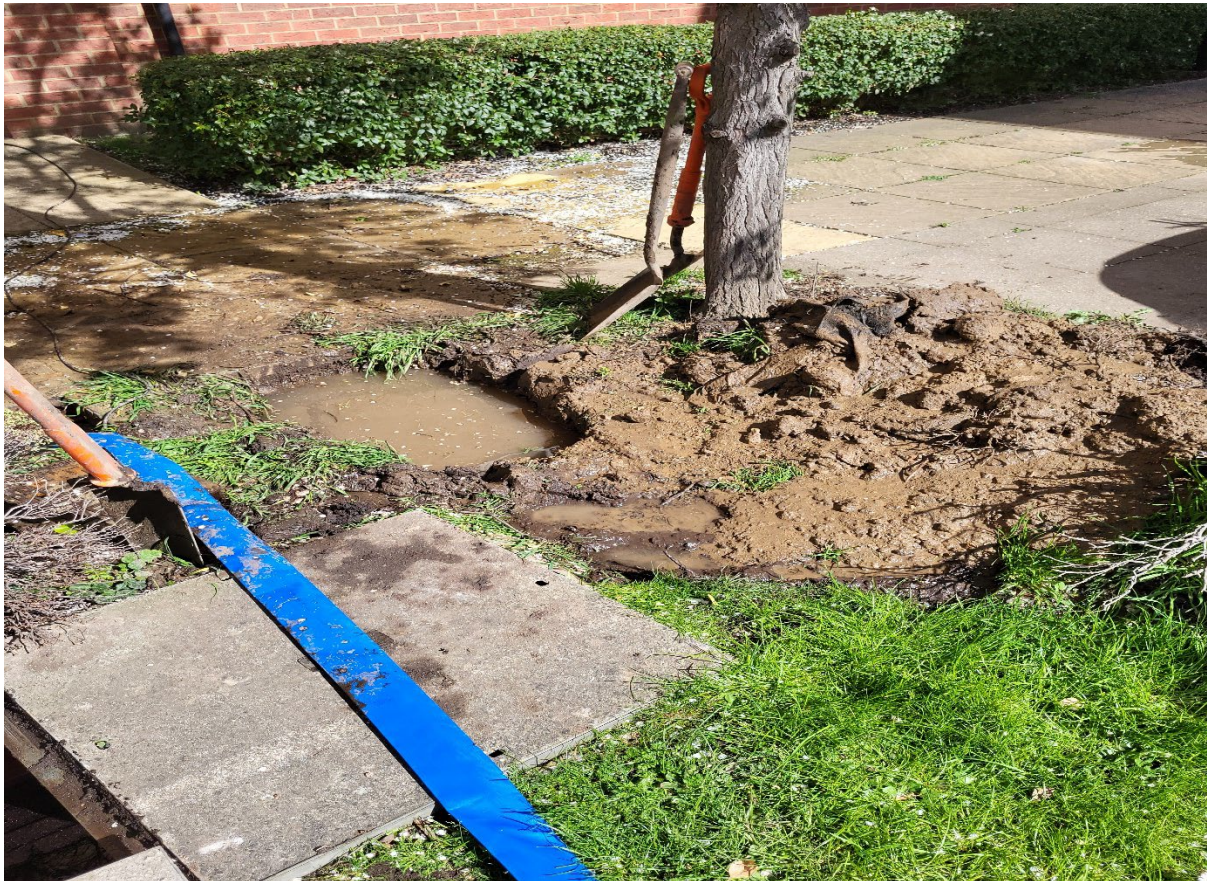
Attended site for flooded path/gardens
