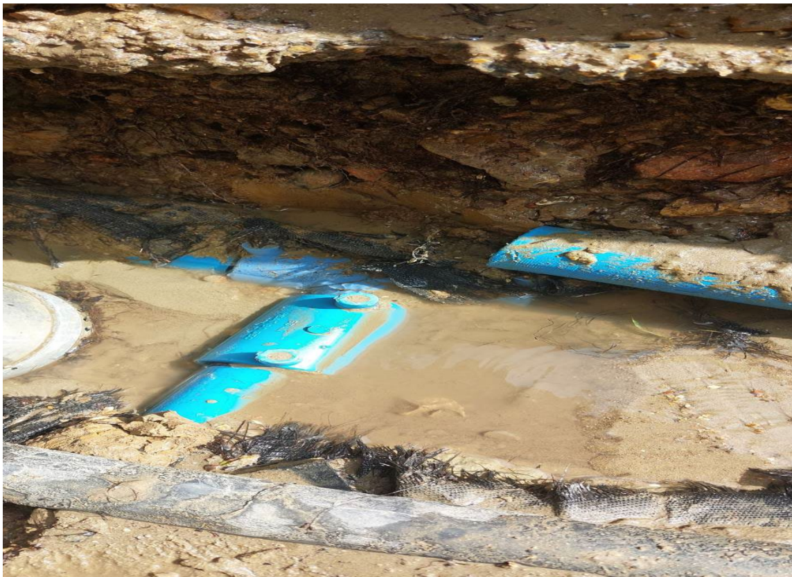
Excavated and found the damaged cold water supply pipe
