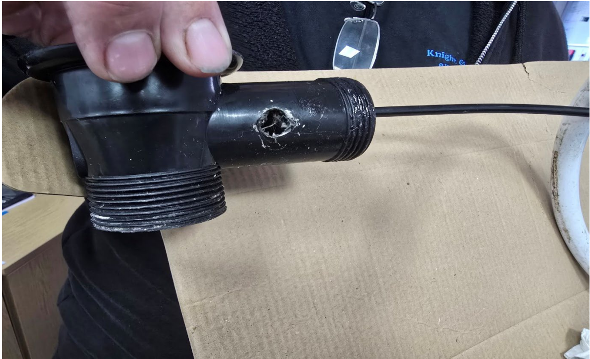
Removed old plug waste and confirmed a hole exists causing the leaks
