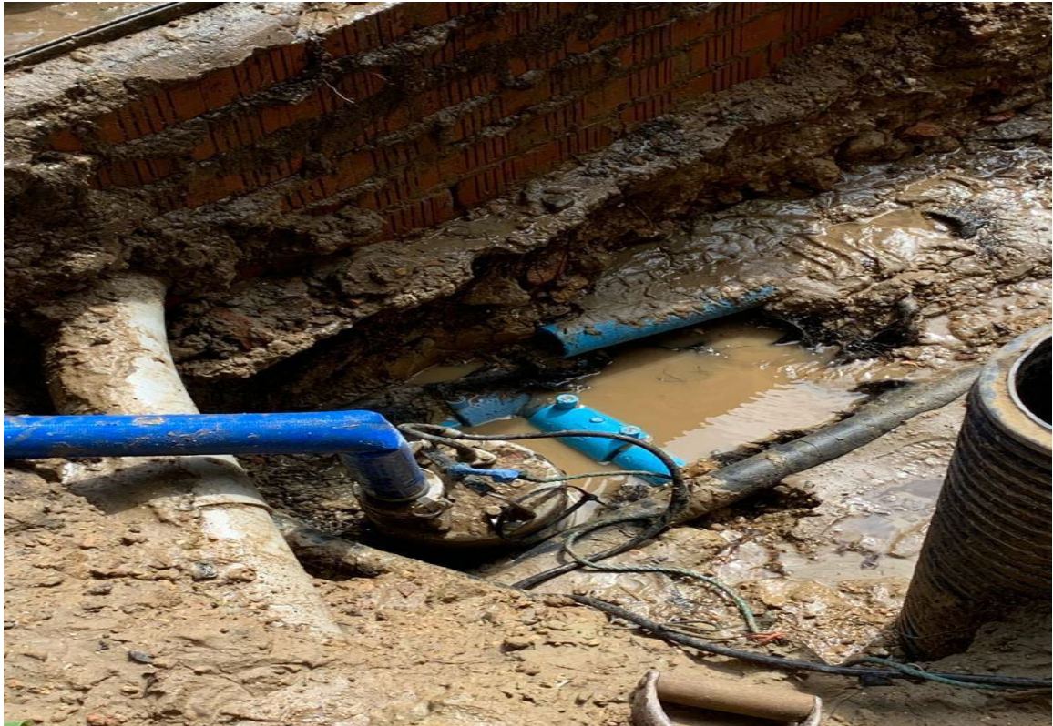
Defective and damaged main water supply pipe exposed
