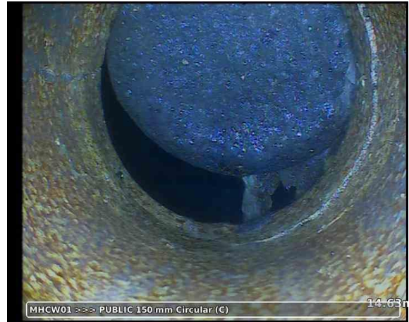
20260203-131500-snap0013.jpg, 00:06:06, 14.63 m Finish node, major connection without manhole, reference: PUBLIC
