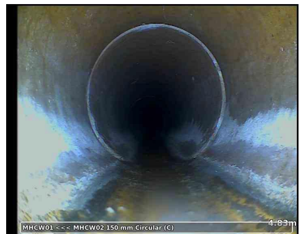
20260203-130158-snap0007.jpg, 00:03:47, 4.83 m Crack, longitudinal at joint at 12 o'clock
