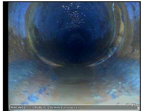
20260203-131500-snap0007.jpg, 00:02:20, 7.45 m Fracture, circumferential at joint from 2 o'clock to 5 o'clock
