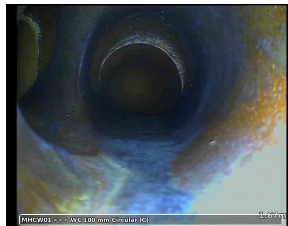
20260203-131157-snap0003.jpg, 00:00:45, 1.67 m Junction at 10 o'clock, 100mm dia
