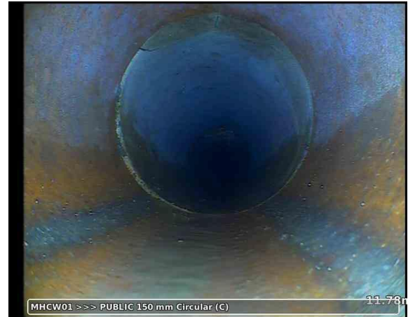
20260203-131500-snap0009.jpg, 00:03:35, 11.78 m Fracture, circumferential at joint from 10 o'clock to 12 o'clock
