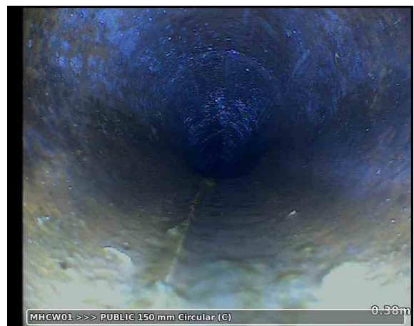
20260203-131500-snap0003.jpg, 00:01:00, 0.38 m Cured-in-place lining ends at this point
