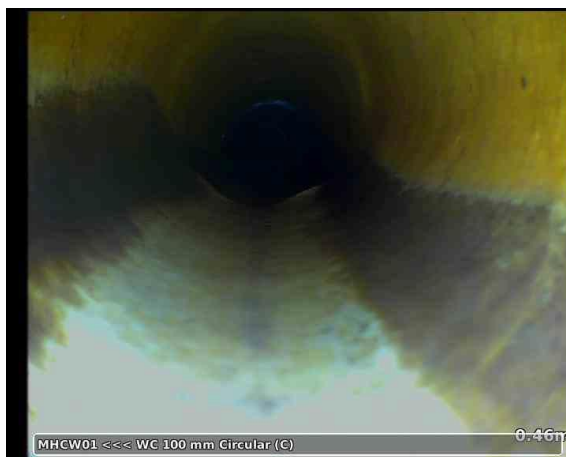
20260203-131157-snap0002.jpg, 00:00:16, 0.46 m Line deviates up
