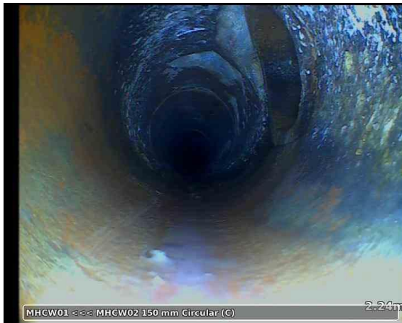
20260203-130158-snap0004.jpg, 00:02:17, 2.20 m Connection other than junction at 3 o'clock, 100mm dia
