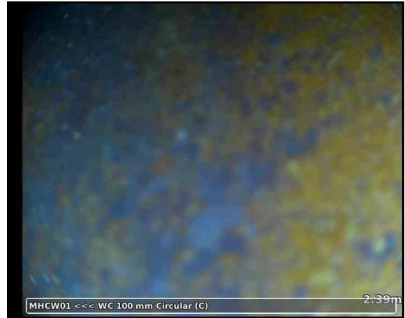
20260203-131157-snap0005.jpg, 00:01:12, 2.39 m Line deviates up
