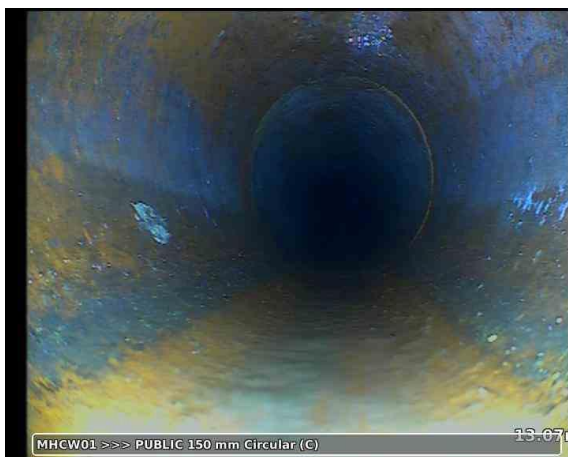
20260203-131500-snap0010.jpg, 00:04:12, 13.07 m Fracture, circumferential at joint from 12 o'clock to 1 o'clock
