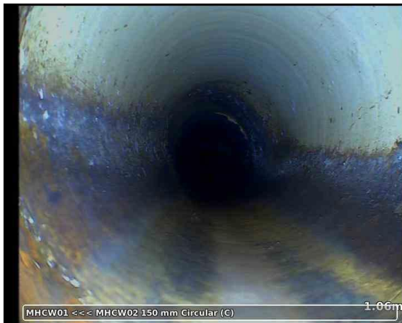
20260203-130158-snap0002.jpg, 00:01:31, 1.06 m Cured-in-place lining ends at this point
