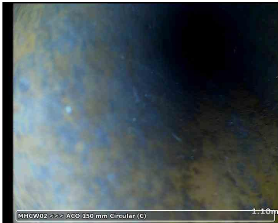
20260203-133243-snap0004.jpg, 00:00:52, 1.10 m Line deviates up
