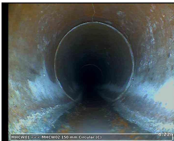
20260203-130158-snap0006.jpg, 00:03:20, 4.22 m Crack, longitudinal at joint at 12 o'clock
