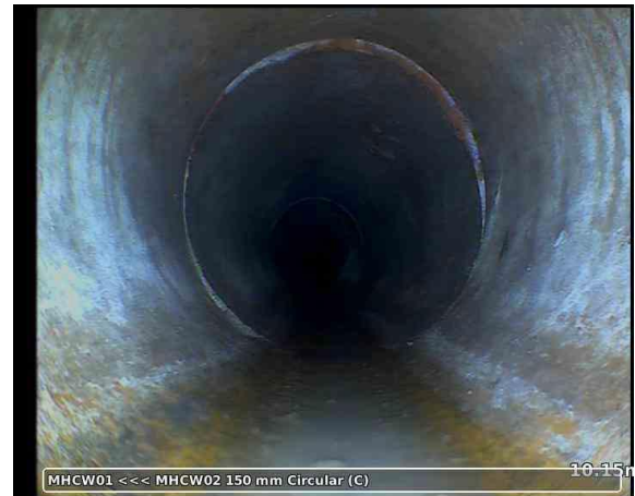
20260203-130158-snap0009.jpg, 00:05:19, 10.15 m Cured-in-place lining ends at this point
