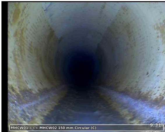
20260203-130158-snap0008.jpg, 00:04:51, 9.31 m Cured-in-place lining ends at this point
