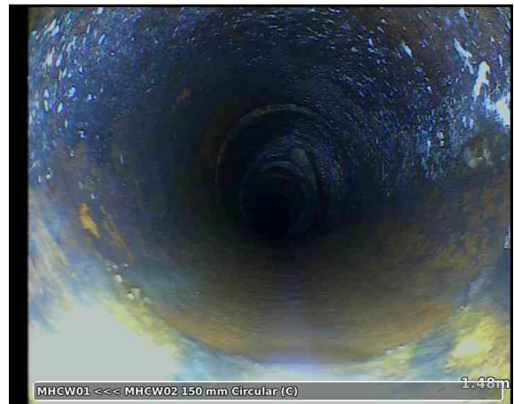
20260203-130158-snap0003.jpg, 00:01:53, 1.48 m Cured-in-place lining ends at this point
