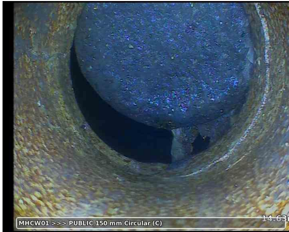
20260203-131500-snap0012.jpg, 00:05:29, 14.63 m General remark, SEWER FLAP
