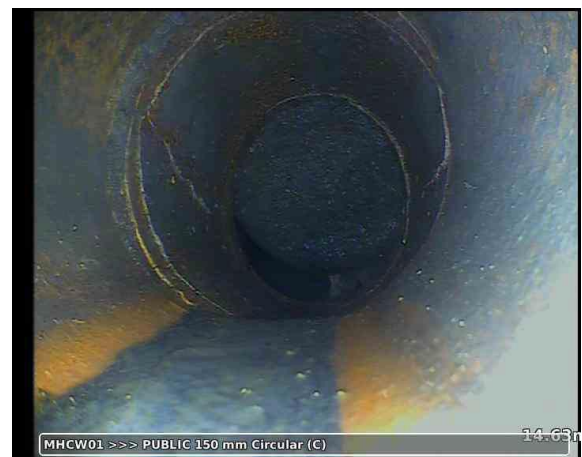
20260203-131500-snap0011.jpg, 00:05:07, 14.63 m Fracture, spiral at joint from 12 o'clock to 12 o'clock
