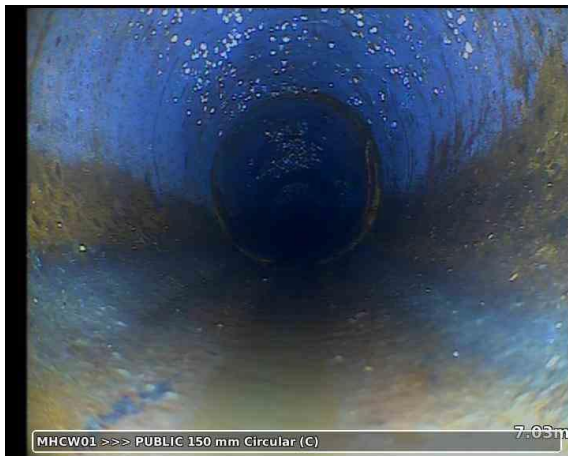
20260203-131500-snap0006.jpg, 00:02:03, 7.03 m Cured-in-place lining ends at this point
