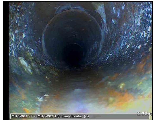
20260203-130158-snap0005.jpg, 00:02:52, 2.58 m Cracks, spiral at joint from 11 o'clock to 12 o'clock
