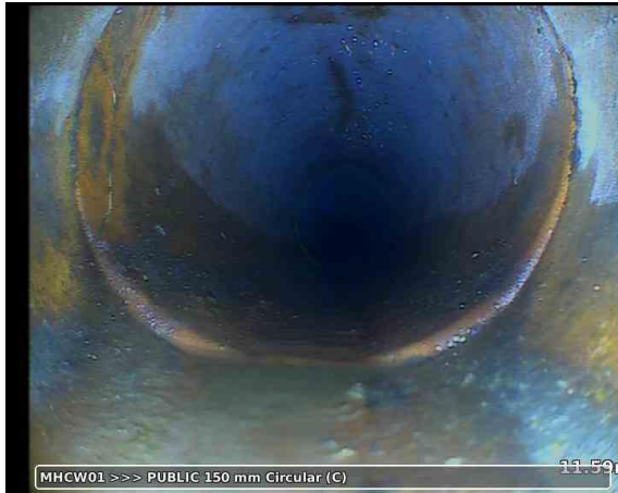
20260203-131500-snap0008.jpg, 00:03:11, 11.59 m Crack, circumferential at joint from 8 o'clock to 10 o'clock
