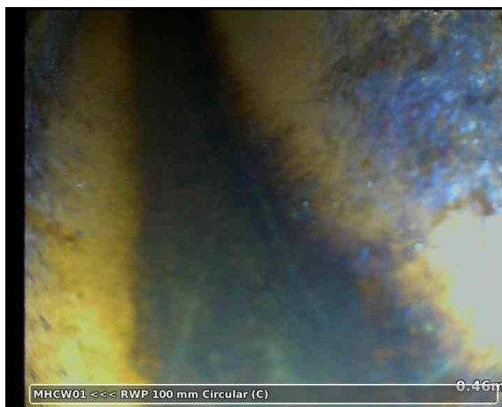
20260203-130931-snap0002.jpg, 00:00:17, 0.46 m Line deviates up
