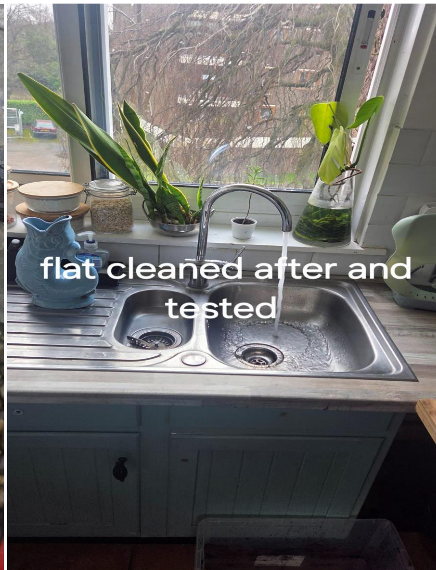
picote machine showing sludge on cable
