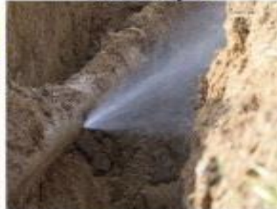
Burst - Leaking Pipe
